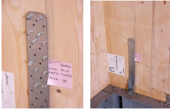
Figure 12: Hold-down failure after Nocera Umbra 1.20g
